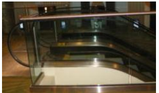
TOP OF ESCALATORS
