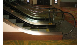
BOTTOM OF ESCALATORS
